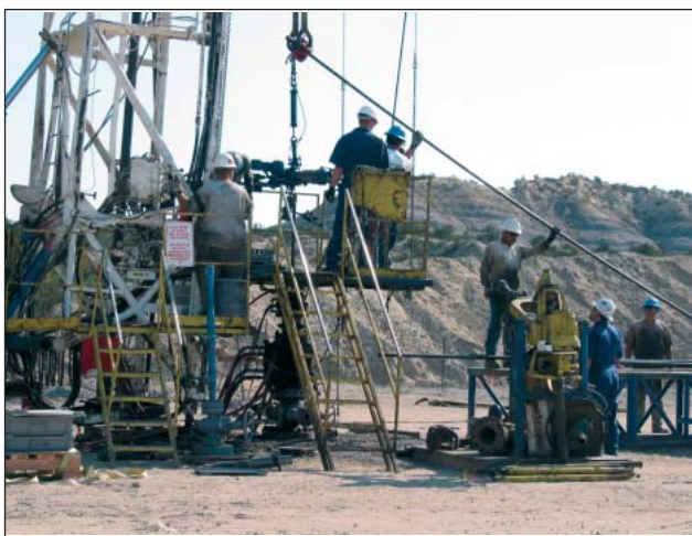
Figure 3 A work-over rig deploying the production tubing to which the downhole receiver array is attached.
