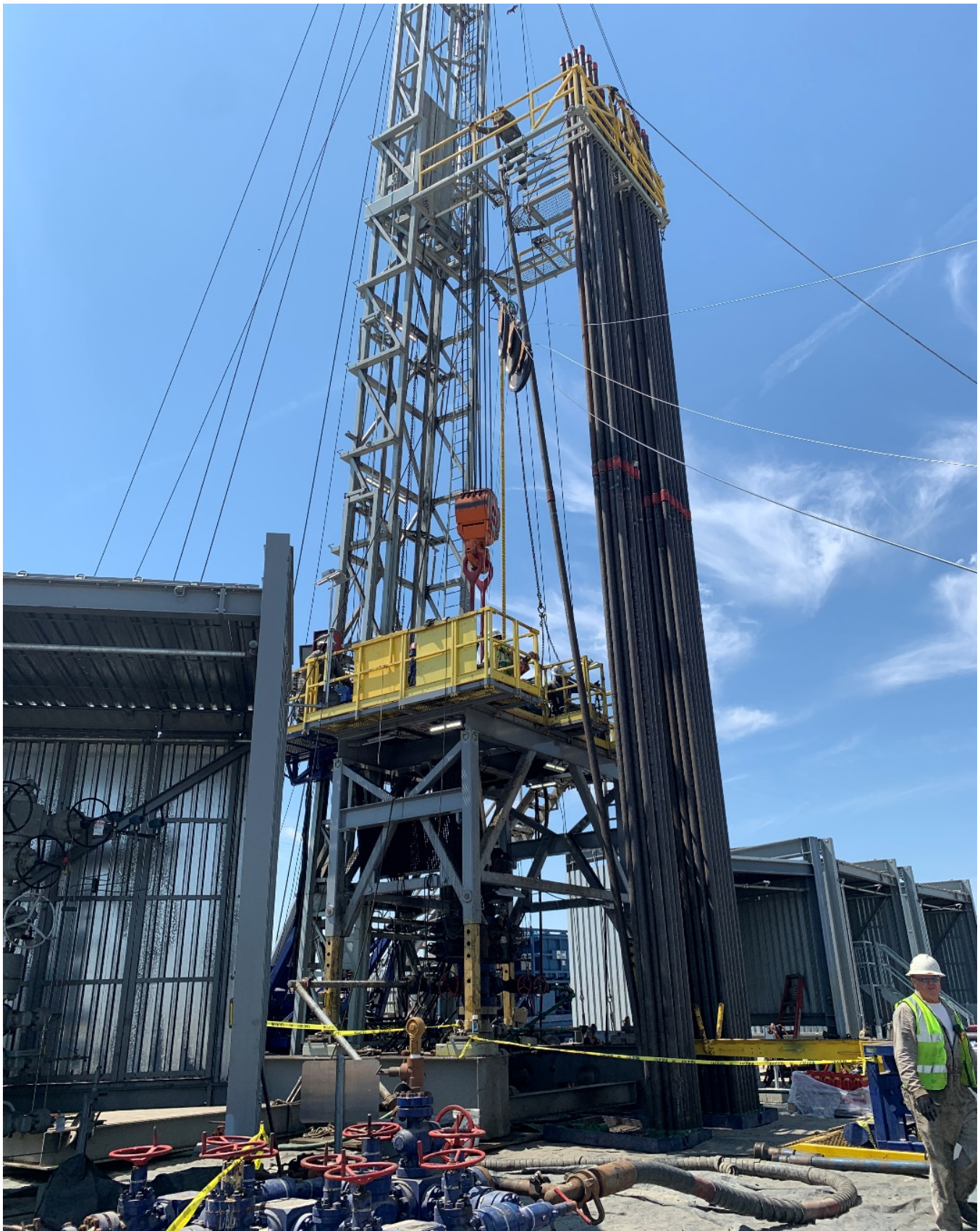
Figure 5. The drilling rig at the McDonald Island UGS in the process to deploy the 4.5" OD production tubulars into the well. The Paulsson fiber optic sensors are enclosed in the 1/4" stainless tubing shown on the right hand of the figure. This 1/4" tube with fiber is mounted to the 4.5" production tubing.
