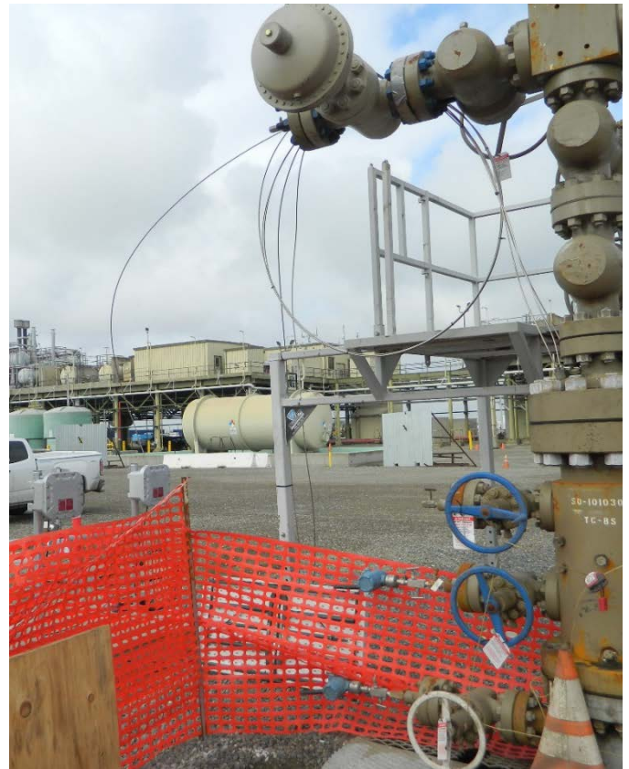
Figure 4. Showing fiber optic cable spliced connection boxes at surface immediately following installation.
