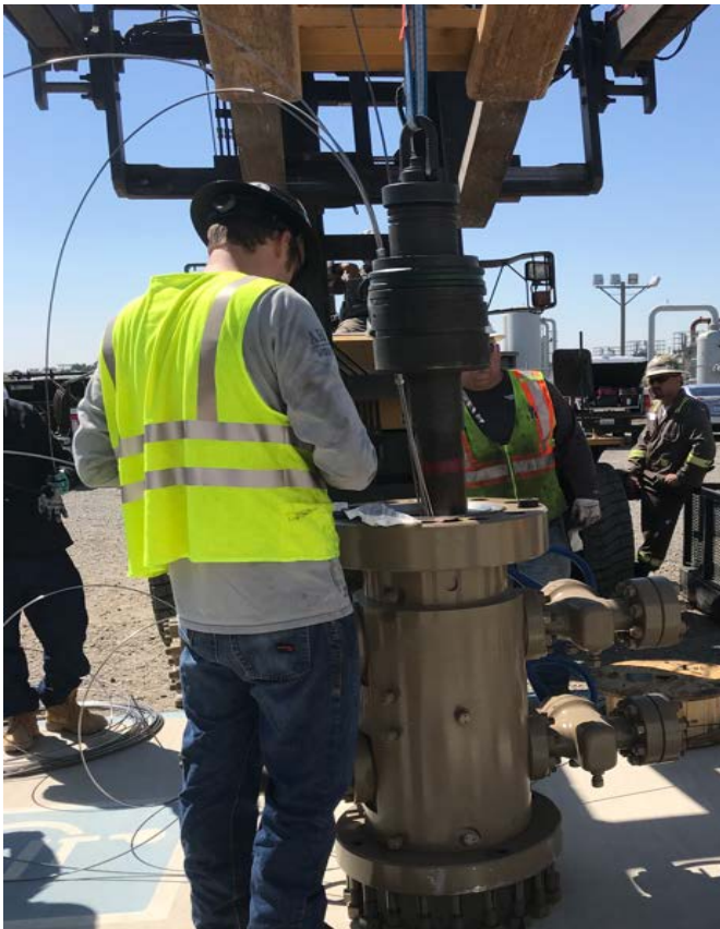
Figure 3. Showing Internal Porting in the wellhead that allows fiber optic cable to enter the well.
